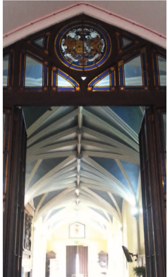
Fig. 9. Wyatt's entrance vestibule and screen, Cobham Hall. (Author, with thanks to Cobham Hall School)
