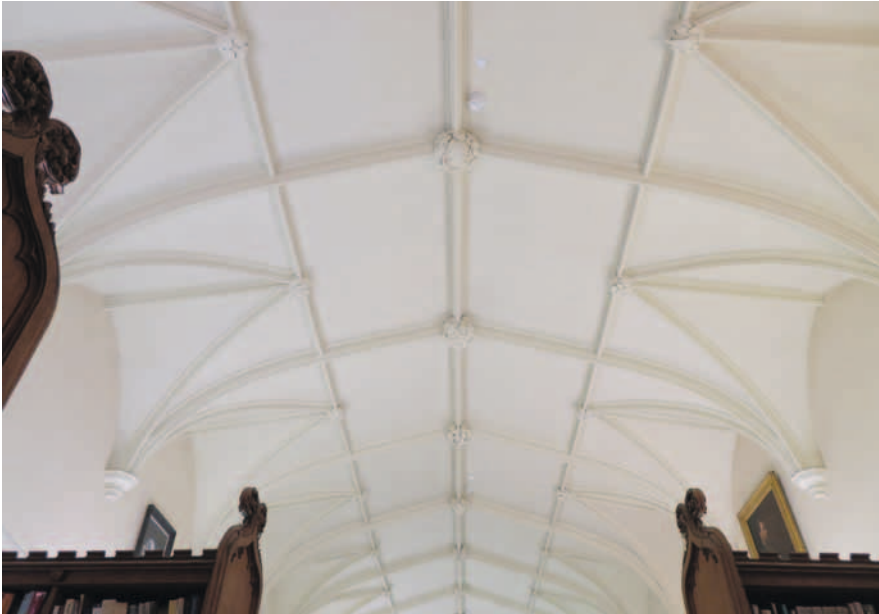
Fig. 20. The ceiling of Balliol College, Oxford, executed in 1794 by Bernato Bernasconi for James Wyatt. (Author, by kind permission of The Master and Fellows of Balliol College, Oxford )
