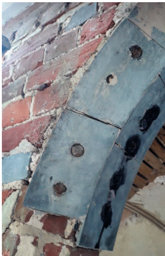
Fig. 15. Slate slips around a window architrave at Cobham Dairy before restoration, showing the bedding and fixing methods. (Author)
