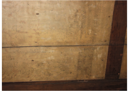
Fig. 9. Tower Green No. 5, fictive panelling, detail of oak graining. ( Historic Royal Palaces )
