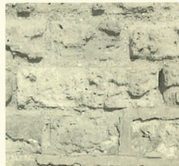
WHAT REPOINTING WITH A STRONG CEMENT MORTAR CAN DO TO A BRICK WALL
