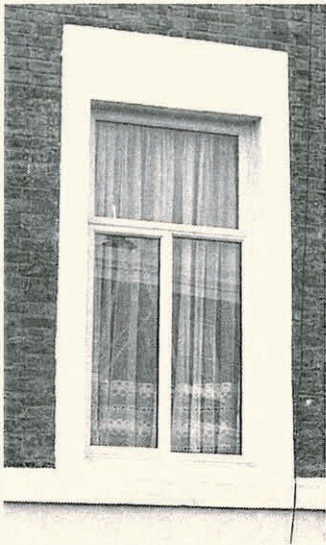
A PARTICULARLY UNSYMPATHETIC WINDOW REPLACEMENT AND LOSS OF SURROUNDING MOULDINGS.
