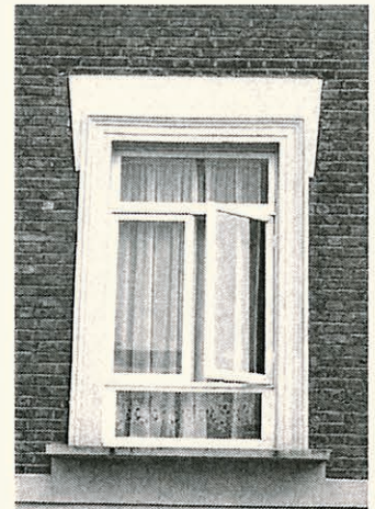
THIS UPVC REPLACEMENT MAKES NO ATTEMPT EVEN TO MIMIC A SASH.
