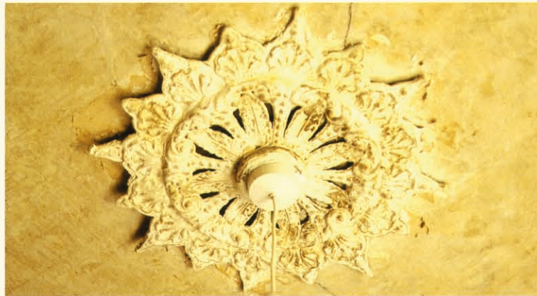
A PAPIER MACHE CEILING ROSE DISCOVERED AS A RESULT OF PAINT STRIPPING
