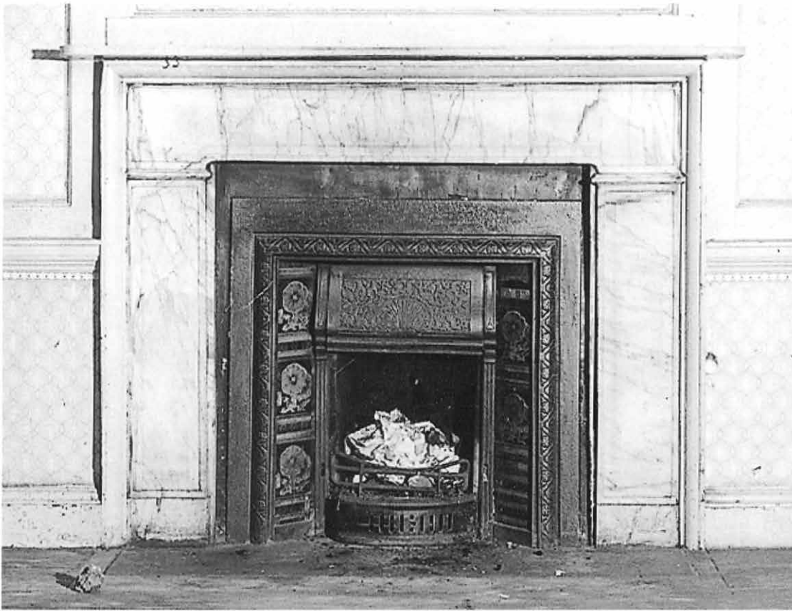
7. GREAT YARMOUTH DRURY HOUSE, SOUTH QUAY, parlour chimneypiece composed of moulded marble jambs and entablature set directly into the panelling (photo NMR: ref. BB67/2278)
