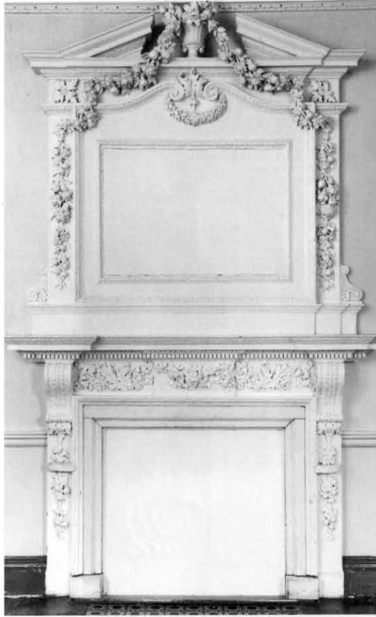
23. YORK, BOOTHAM, 1st floor front room, a continued chimneypiece designed by John Carr (photo NMR: ref YC1633)
